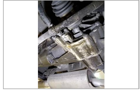
Oil Leaks 1 - Image 1 of 2
